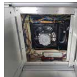
A5. Condenser compartment
